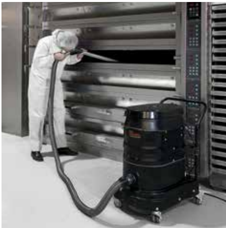
R01 A024 for suctioning furnaces
